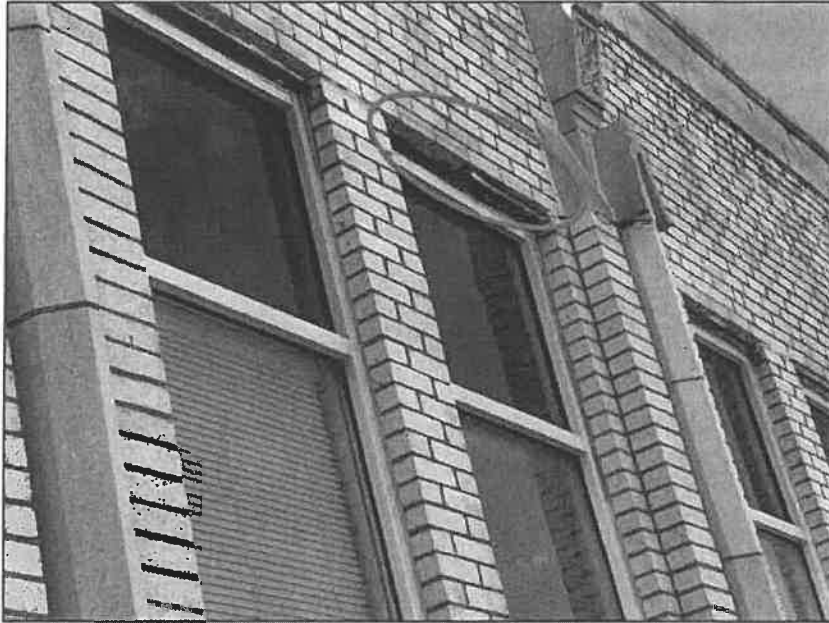
Photograph 3 - Unsupported Brick above 7 th Floor Window
