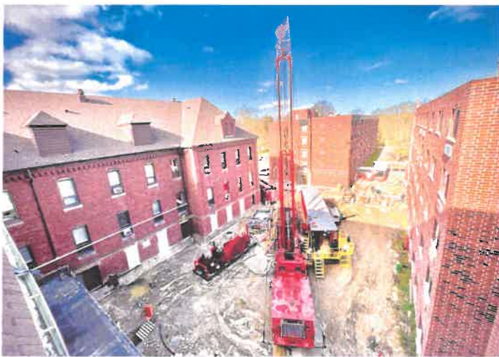
The Well Done Foundation adopted this well from the State of Ohio and plugged it on behalf of the property owner.
