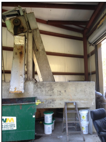
Mechanical Bar Screen to be Replaced
