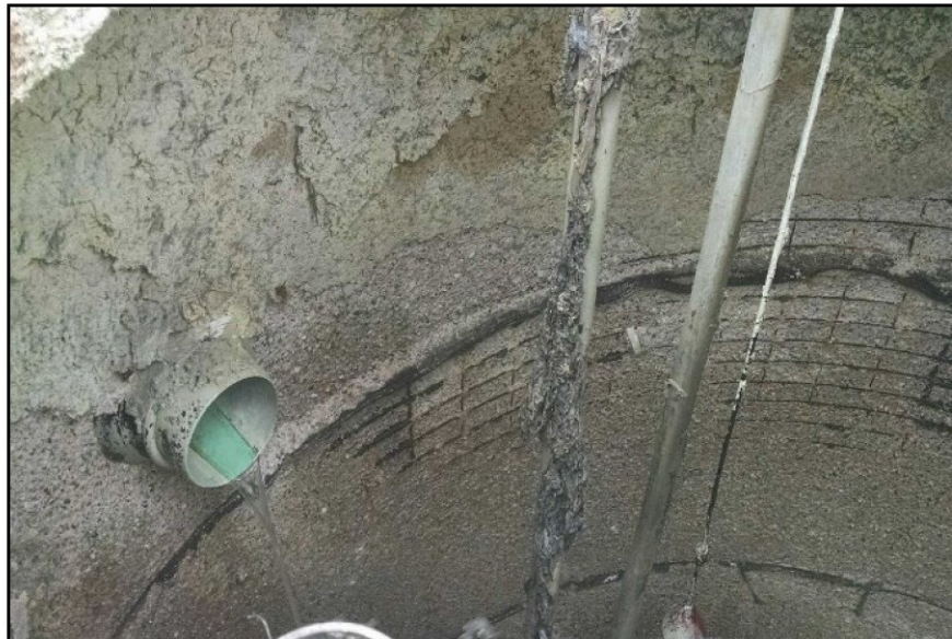
Deteriorated Concrete at Phase II Pump Station Wet Well
