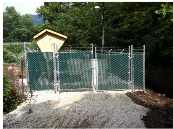
After: Upper Drive Lift Station
