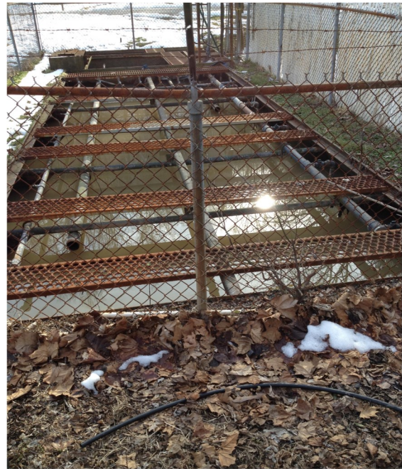
Failing Package Treatment Plant
