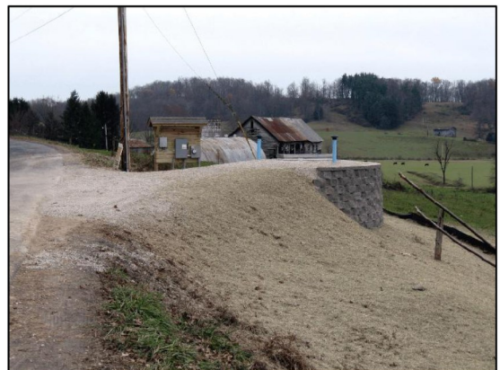
50 GPM Booster Station
