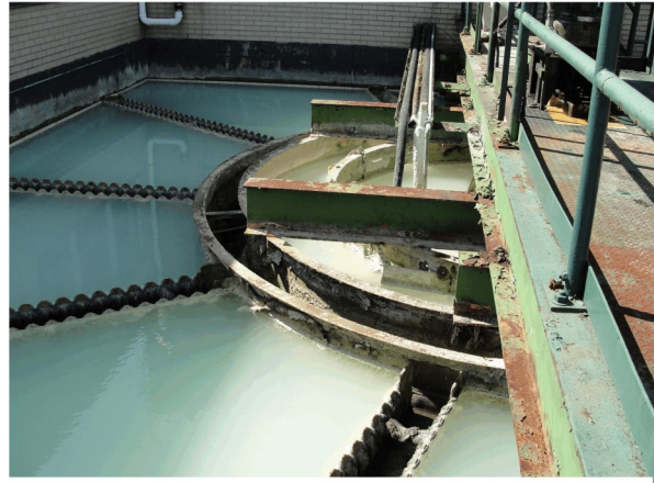
Upflow Clarifier Prior to Replacement
