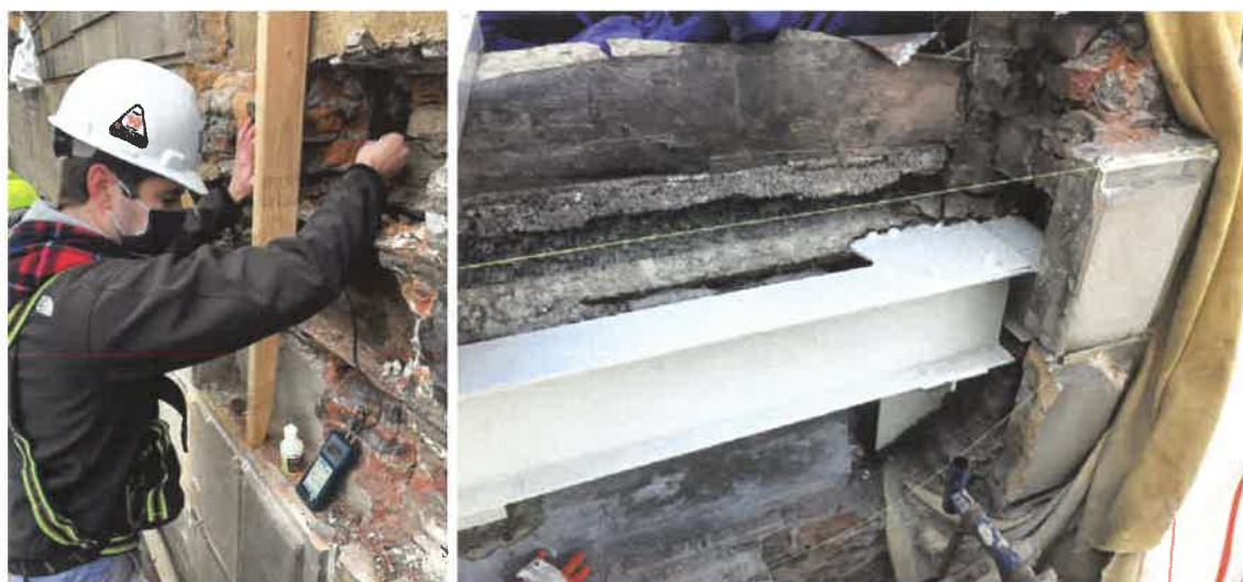
Ultrasonic Pulse Velocity Measurement of Corroded Structural Steel to Evaluate Reduced Capacity [left] and Structural Member Replacement [right]
