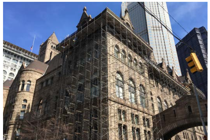
Construction under way, summer 2018—Scaffolding to the eave of the roof line; each week a crane is brought in to unload demo'd materials and load new tile to the top platform.
