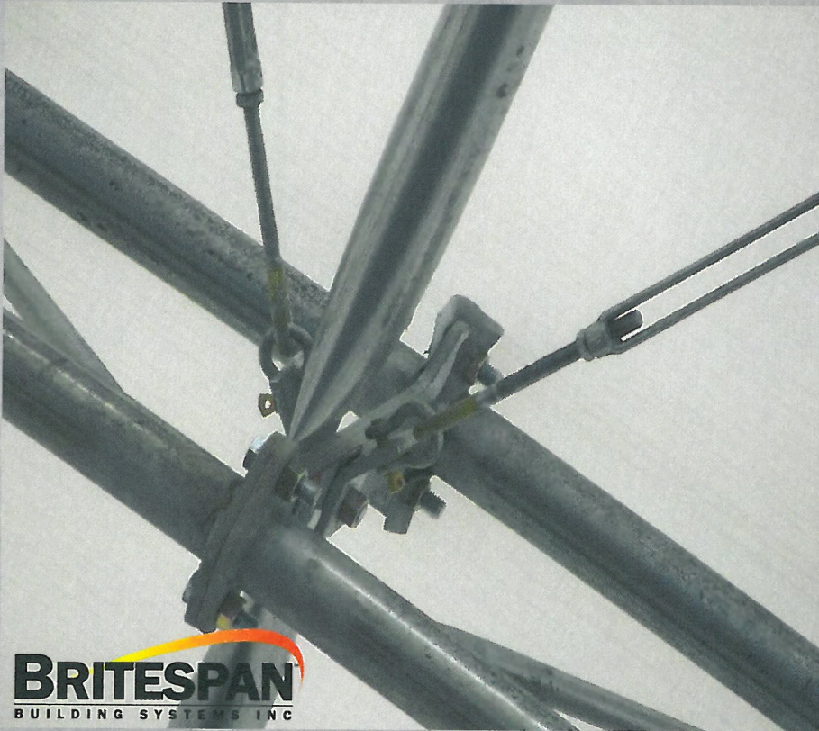
BOLTED AND PINNED TO AN ENGINEERED STRUCTURAL TRUSS MEMBER
