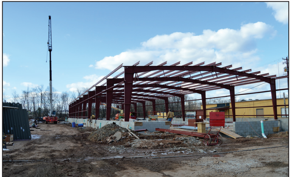
Construction continues at the West Virginia State Agency for Surplus Property. Surplus Property employees are expected to move into the new warehouse and administrative building (above) in April.
