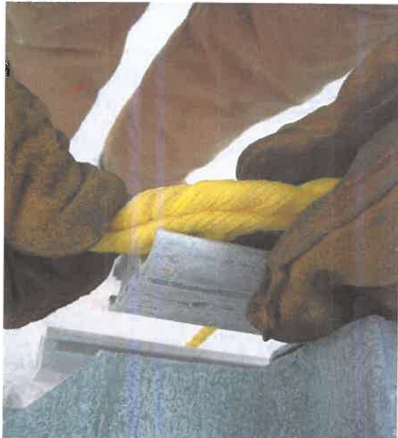
Right Below: Flattening the rope to pull ends out to the side of the Extrusion channel
